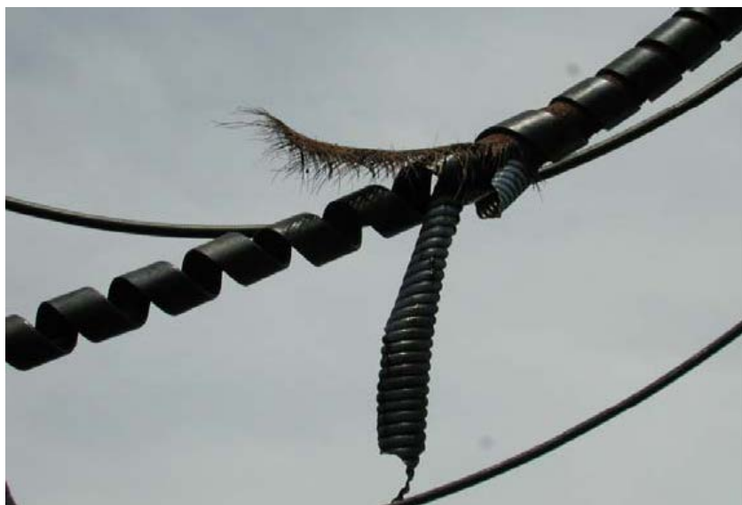
Ruptured chlorine transfer hose with its Teflon inner layer exposed; when the hose burst it ejected pieces of Teflon as well as other components of the hose.
